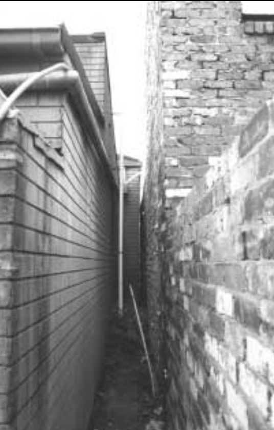
Rear view - new extension to right, obscuring windows in wall to left
